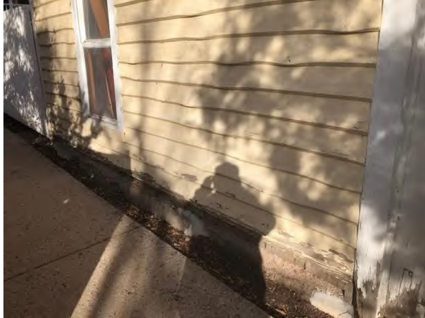
Figure 3 showing deterioration of the miner's cabin at grade.
